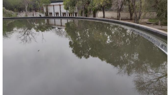
Figure 7: Final Sedimentation Tank
